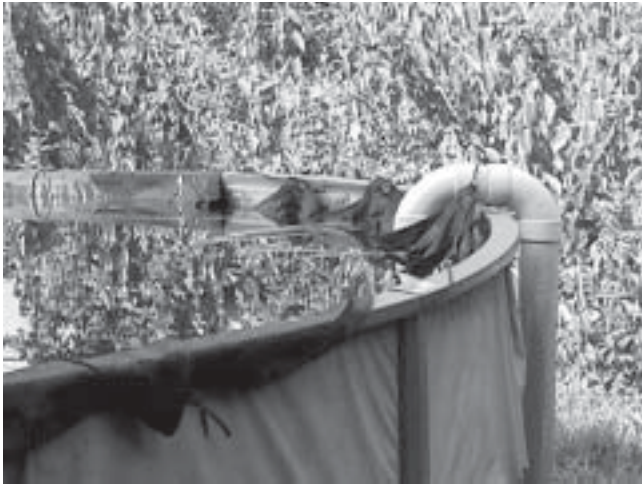
Sagging and broken covers like this one are very common. The storage tank is where water sits the longest, and keeping it covered is important to reducing water contamination.
